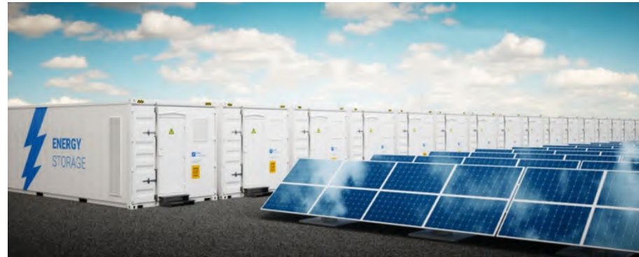
Large scale battery storage system
