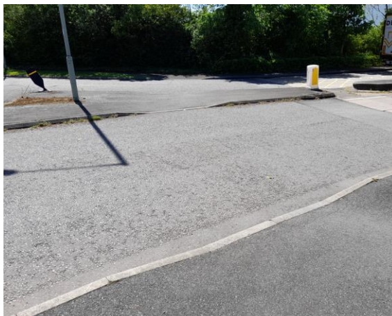
Figure 15 – Absence of tactile paving
