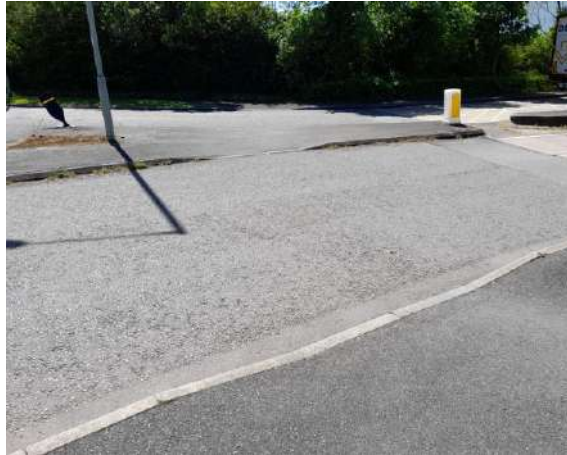
Figure 15 – Absence of tactile paving
