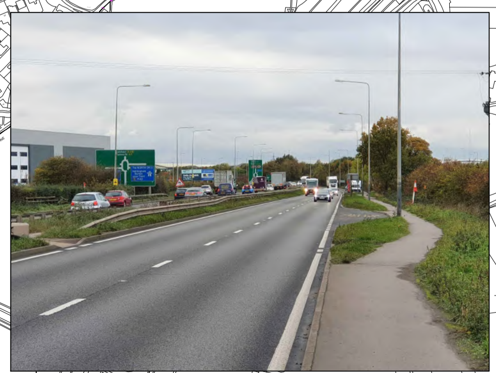
Existing Pinch Point on A5 Pavement / Cycleway at Bus Stop North of A5
