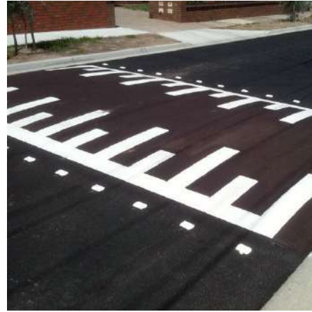
Reflective Road Marking
