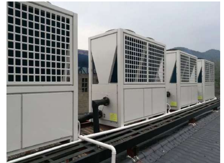
Air source heat pumps
