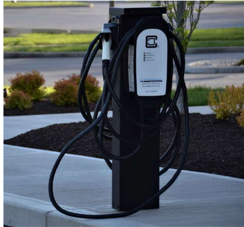
Electric vehicle charging point
