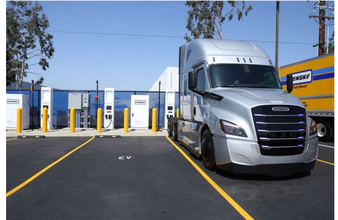
Electric lorry charging points
