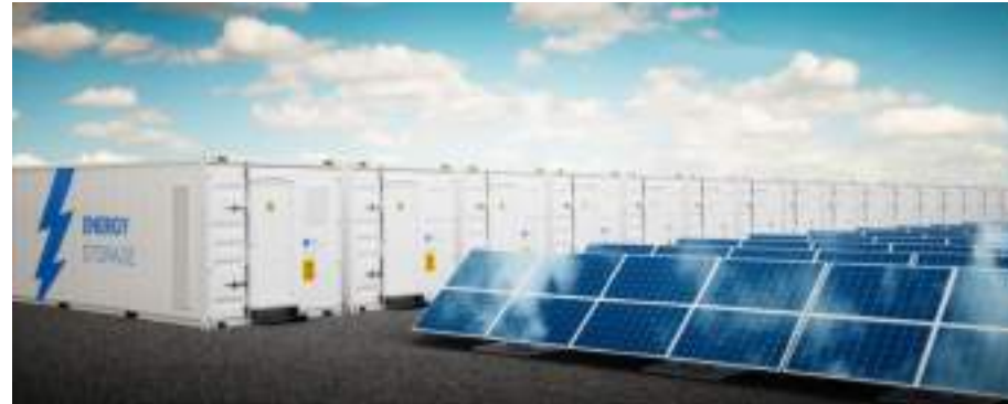
Large scale battery storage system
