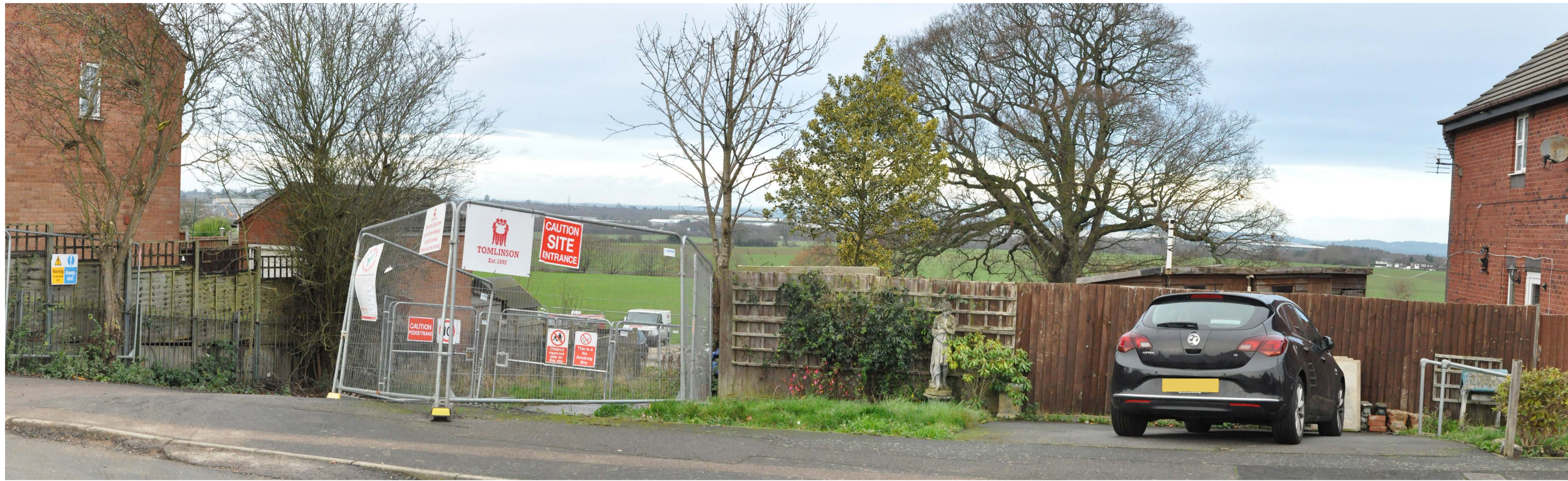
VIEWPOINT: 19 LOOKING WEST TOWARDS THE SITE FROM OFF BIRCHWOOD AVENUE AT ENTRANCE TO TOMLINSON CONSTRUCTION SITE.
