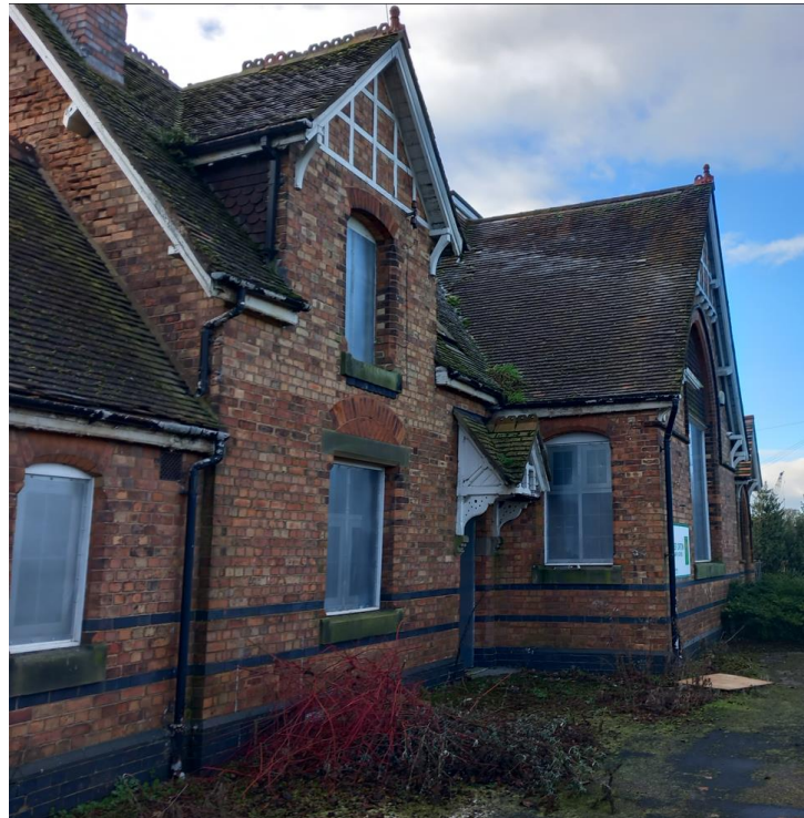
Former Primary School now boarded up, still being entered by vandals causing damage to the interior and roof.
