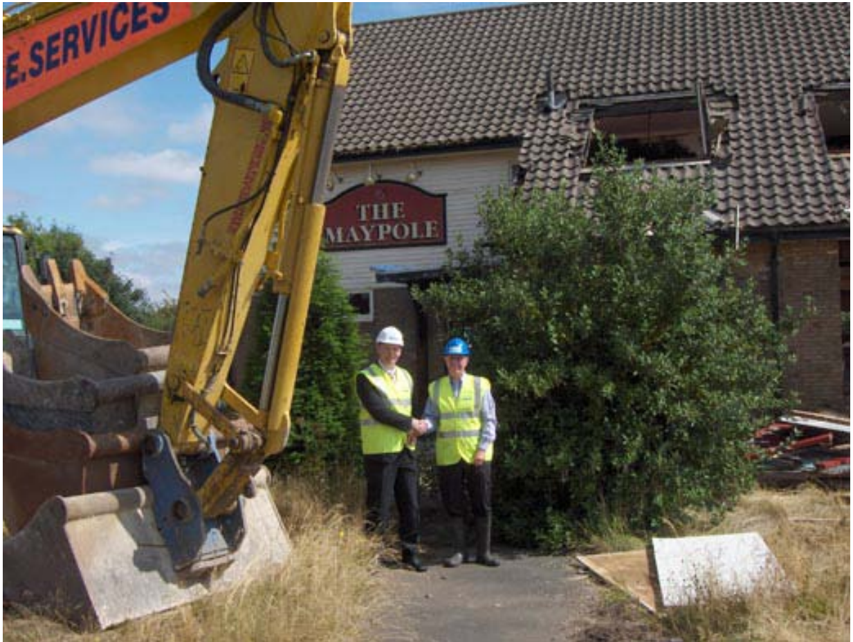
Work commencing on the Colliery Heights, Affordable Housing development at Baddesley Ensor, North Warwickshire.
