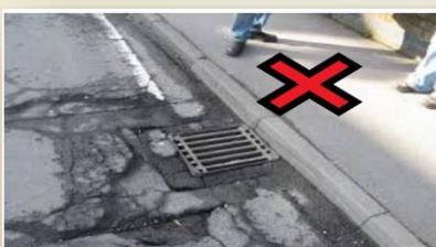
Dangerous and costly "well" drains
