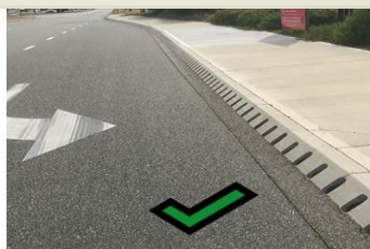
Kerb perforation drains
