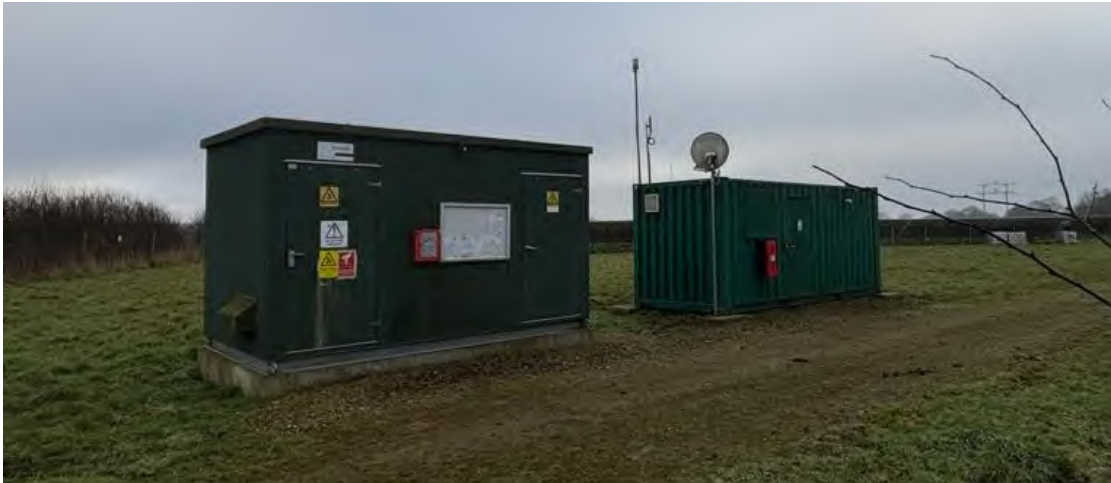
Photo 16: Example of Solar Farm Equipment
