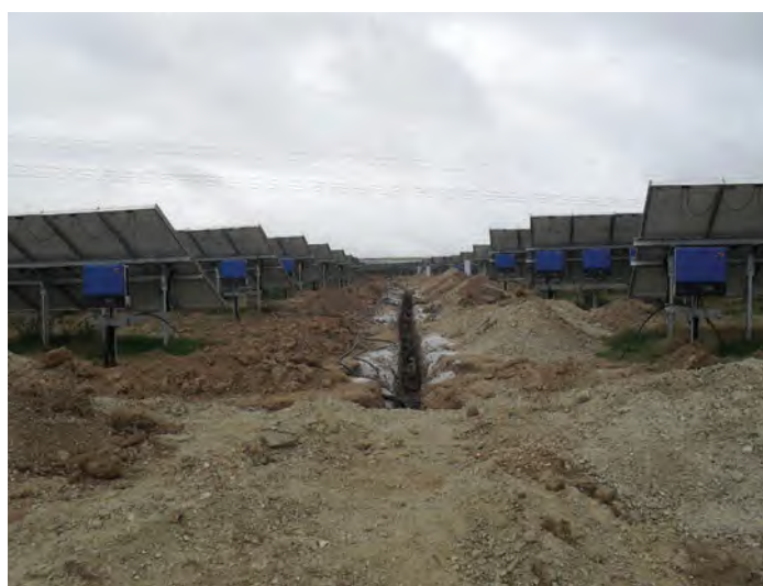
Figure 10 The construction compound associated with the development of the 5MW Trefullock solar farm in Cornwall.
