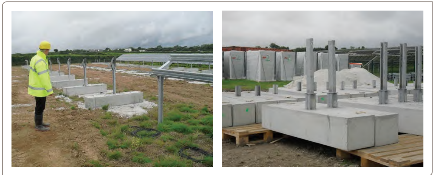
Figure 15 Where there are areas of archaeological interest, and therefore a need to avoid ground disturbance, the use of pre-cast concrete anchors should be considered, as shown here at the 5MW Trefullock solar farm in Cornwall.
