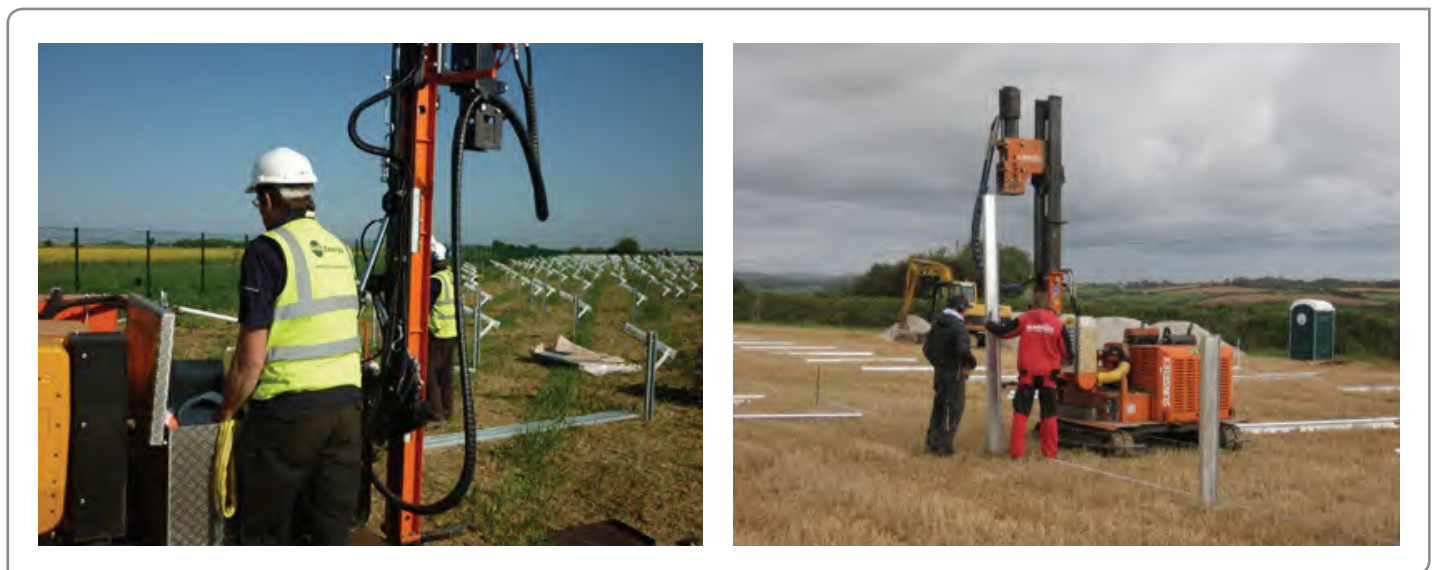
Figure 16 Where pile driven foundations are proposed consideration should be given to the noise impact at nearby sensitive receptors. Difficult ground conditions, such as those encountered at the 1.4MW Wheal Jane solar farm shown here, may also require drilling.
