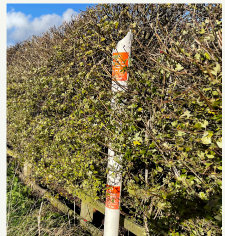
Marker Post identifying Gas Main
