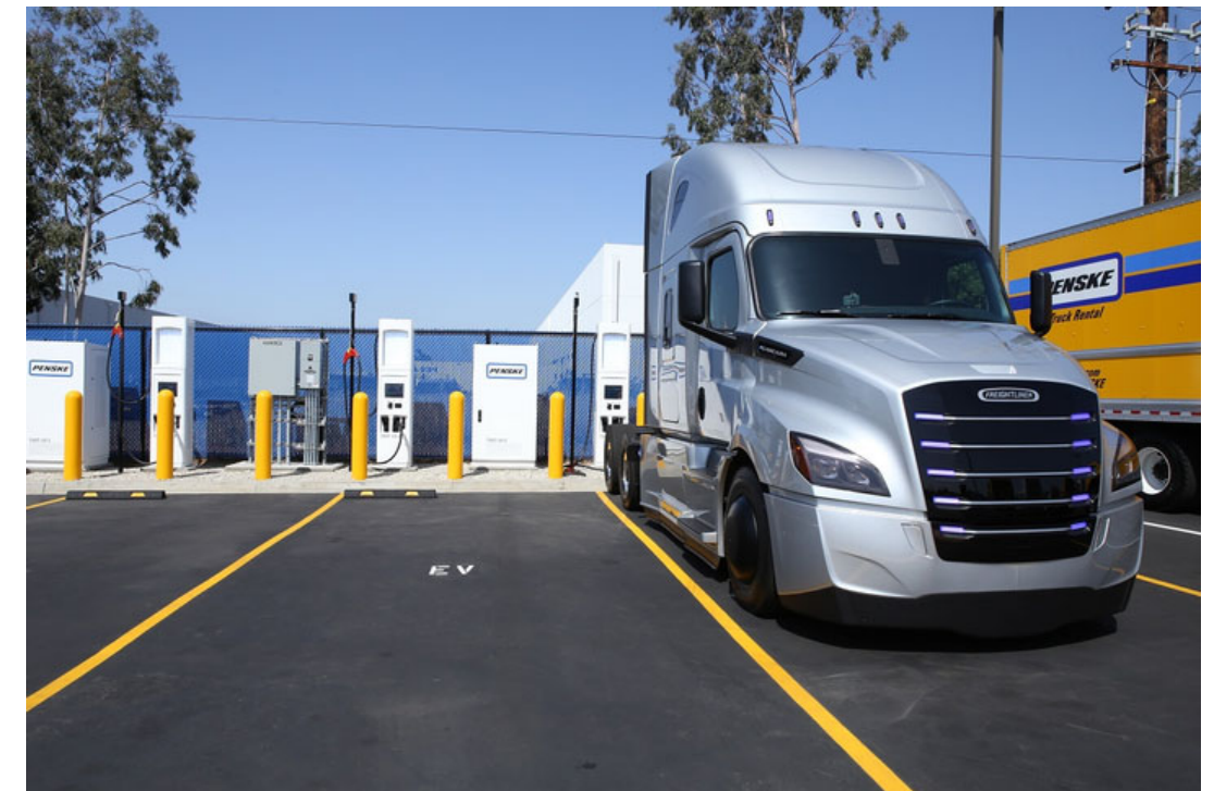
Electric lorry charging points
