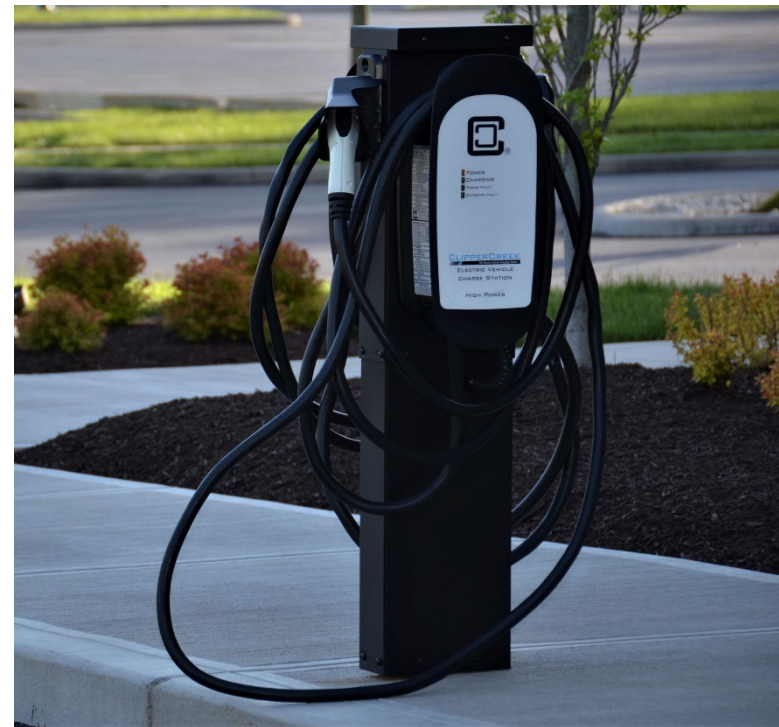
Electric vehicle charging point
