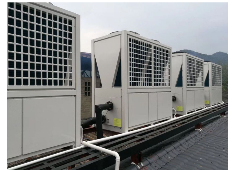
Air source heat pumps
