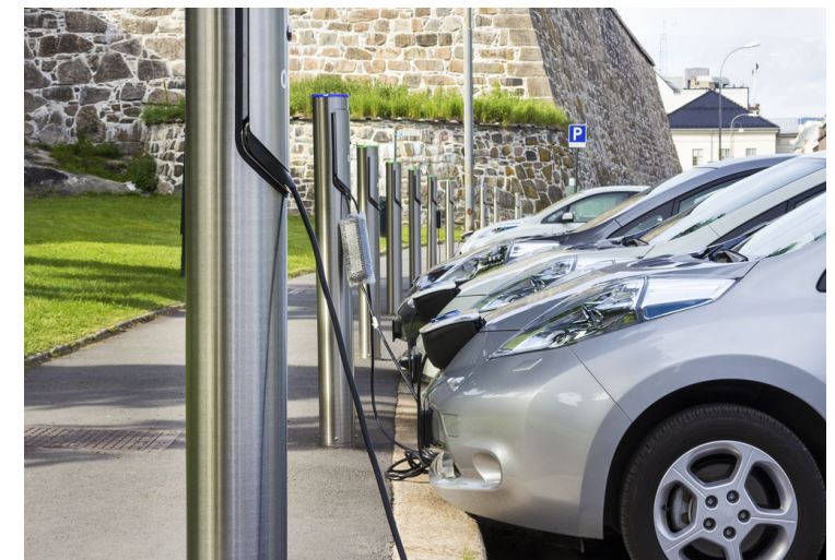
Electric Vehicle charging points
