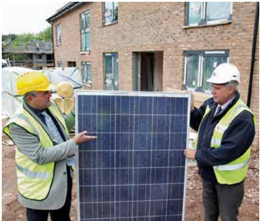
New housing with solar panels
