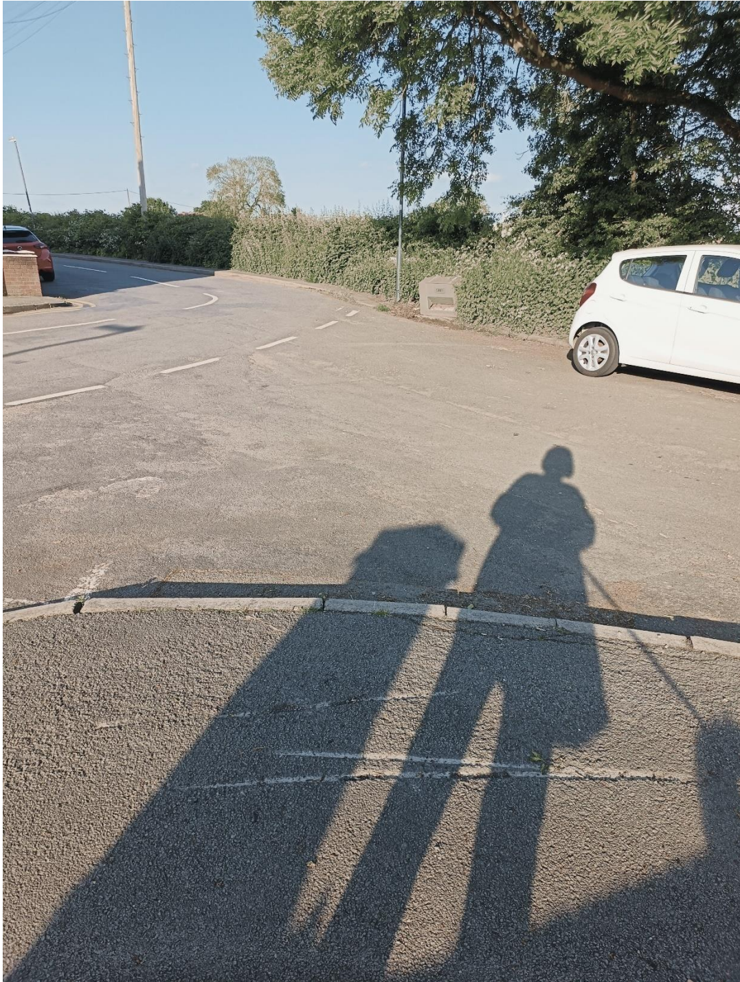
Photograph showing the damage caused to the footway at the junction of Cockspur Street and Green Lane, Birchmoor
