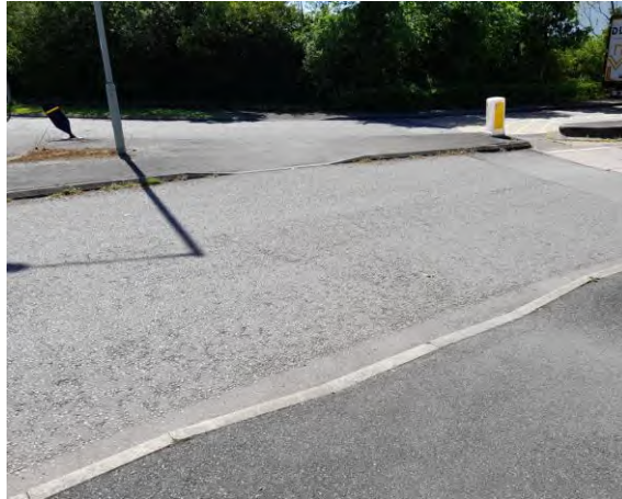
Figure 15 – Absence of tactile paving
