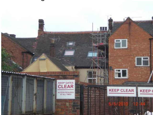
EXAMPLE OF INAPPROPRIATELY LARGE ROOFLIGHTS (REAR OF LONG STREET)
