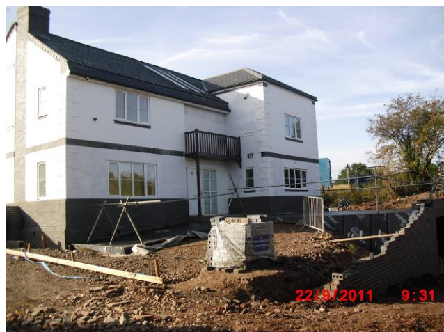
Illustrates the use of incorrect door and glazing in the centre section of the building.
