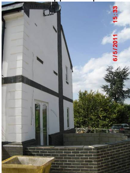
Illustrates the window cills left in situ at first and second floors
