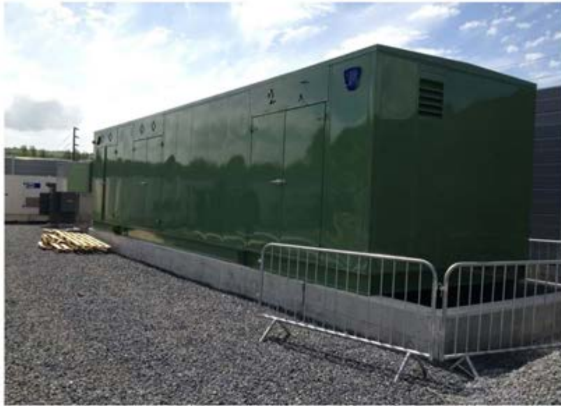
Containerised switch room
