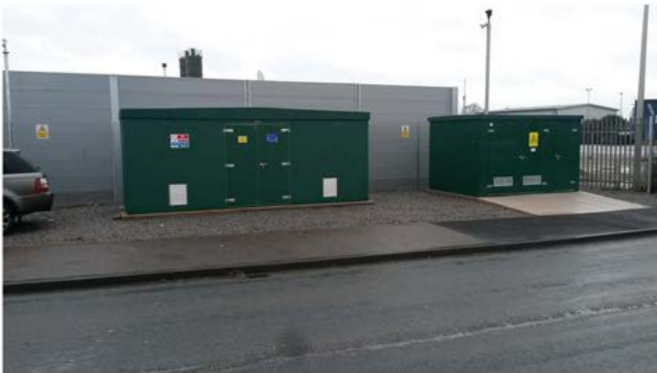
An existing site showing secured compound with internal acoustic fence and external security fence
