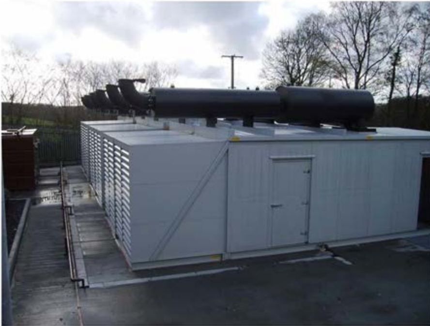
Image of a typical bank of 3 generator canopies (from within an existing compound)
