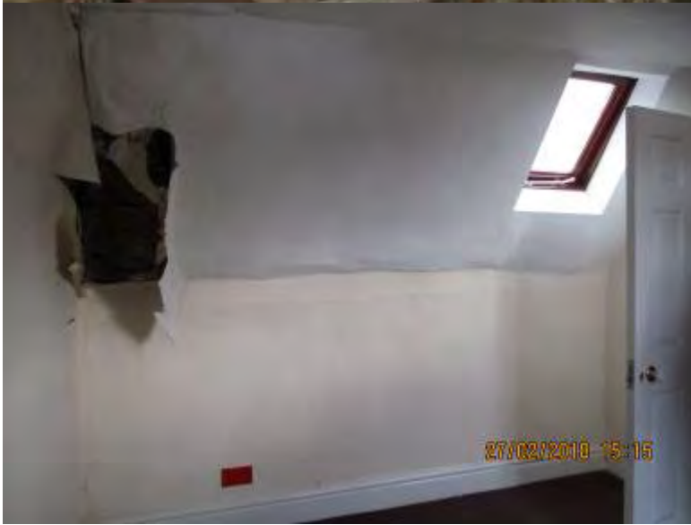
Water ingress – repairs to the ceiling required
