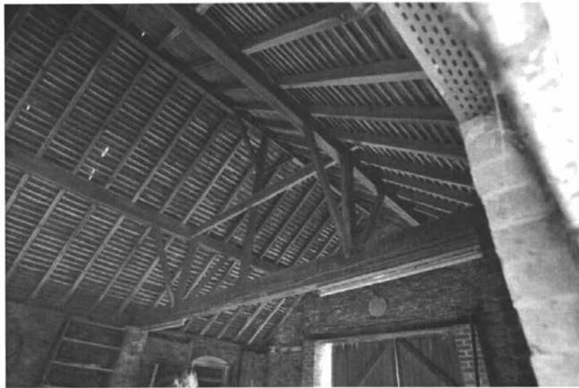
Pl.8: Part of the interior and unusual roof structure of the former Cart Shed.
