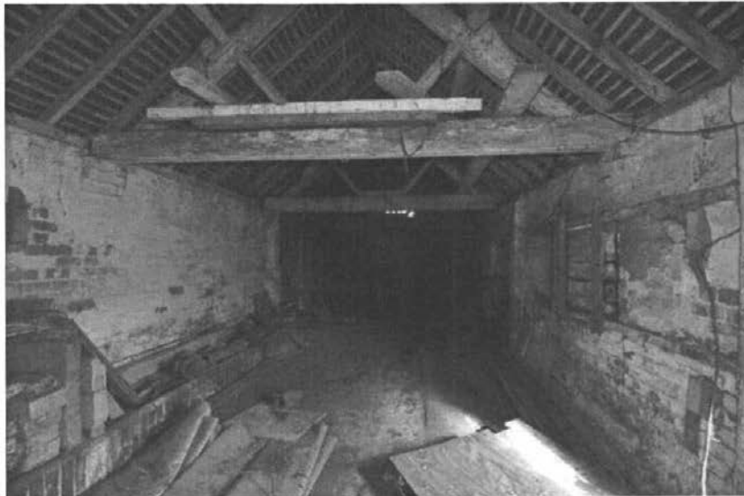
Pl.13: The interior of the South Byre, looking east. Note sliding shutters (right) and trough (left), as well as the design of the roof structure.
