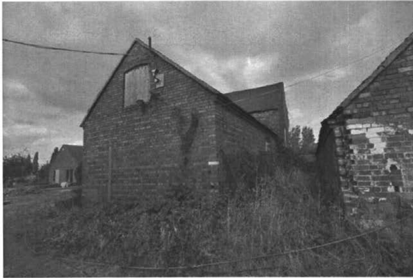
Pl.9: The North Byre (Building C) from the south-west, with the South Byre (Building D) to the right.
