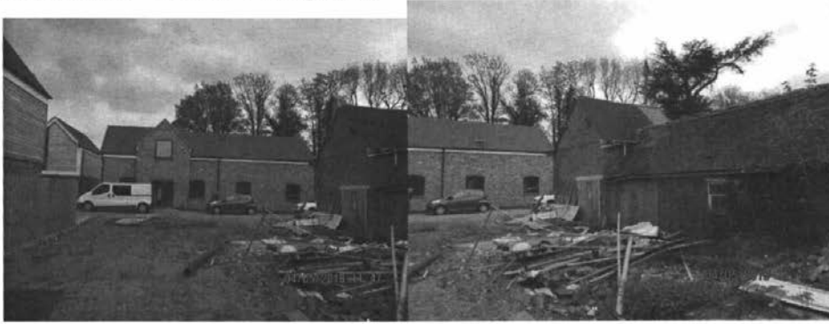
From application site towards No. 1 Hawcutt No.1 Existing building on east side of application site towards No.1
