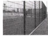
Ball court fencing, weld mesh 3.0m high with lower 1.2m having strengthened rebound mesh panels. Colour green.
