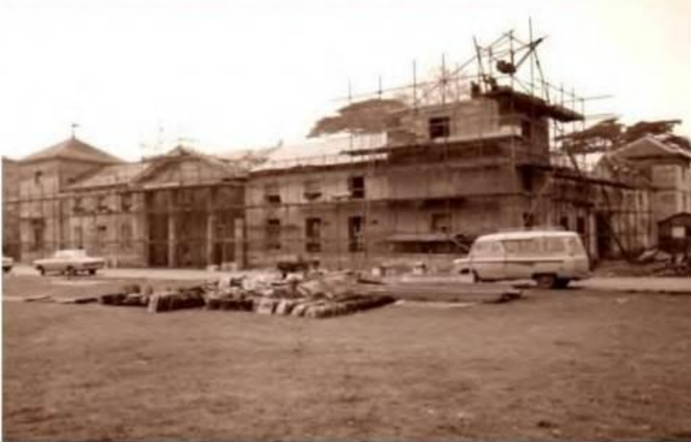
Illustrations from 1970 demonstrating the extent of fabric removal undertaken during the refurbishment works
