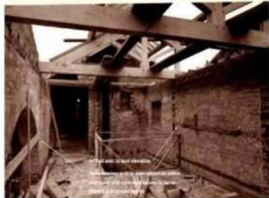
1st floor looking north with the bricked up arch to the east elevation visible on the right and the original arch into the courtyard on the left.
