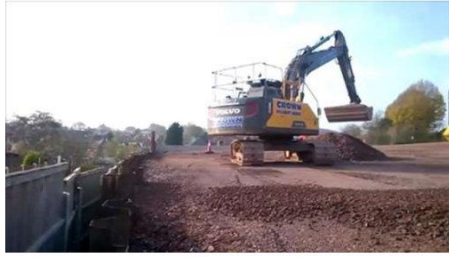
Showing arrival of metal piles, violent installation method and more stone delivered from Tarmac. Also building up of the layers of rock.
