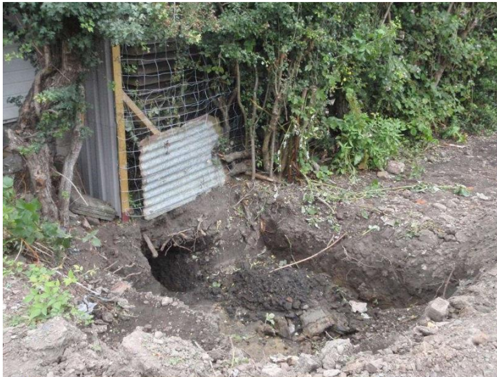
Natural ground height to boundary of 9 Chancery Lane and illegal excavations over boundary line (search for non existent pipes) into 9 Chancery Lane property
