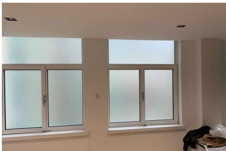
Photographic representation of obscured glazing to the full height of the windows (option 4 only)
