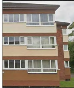
11 - 04 VIEW OF COMPLETED EWI & PITCHED ROOF TO ALEXANDRA COURT, POLESWORTH (Sothern Render System)
