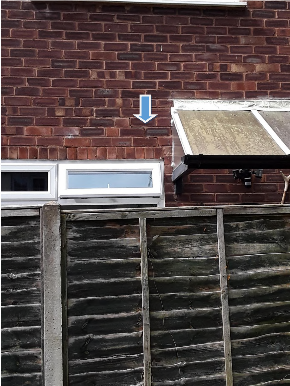
Image 7 – Showing crack in brickwork above the window, cracks in excess of 5mm
