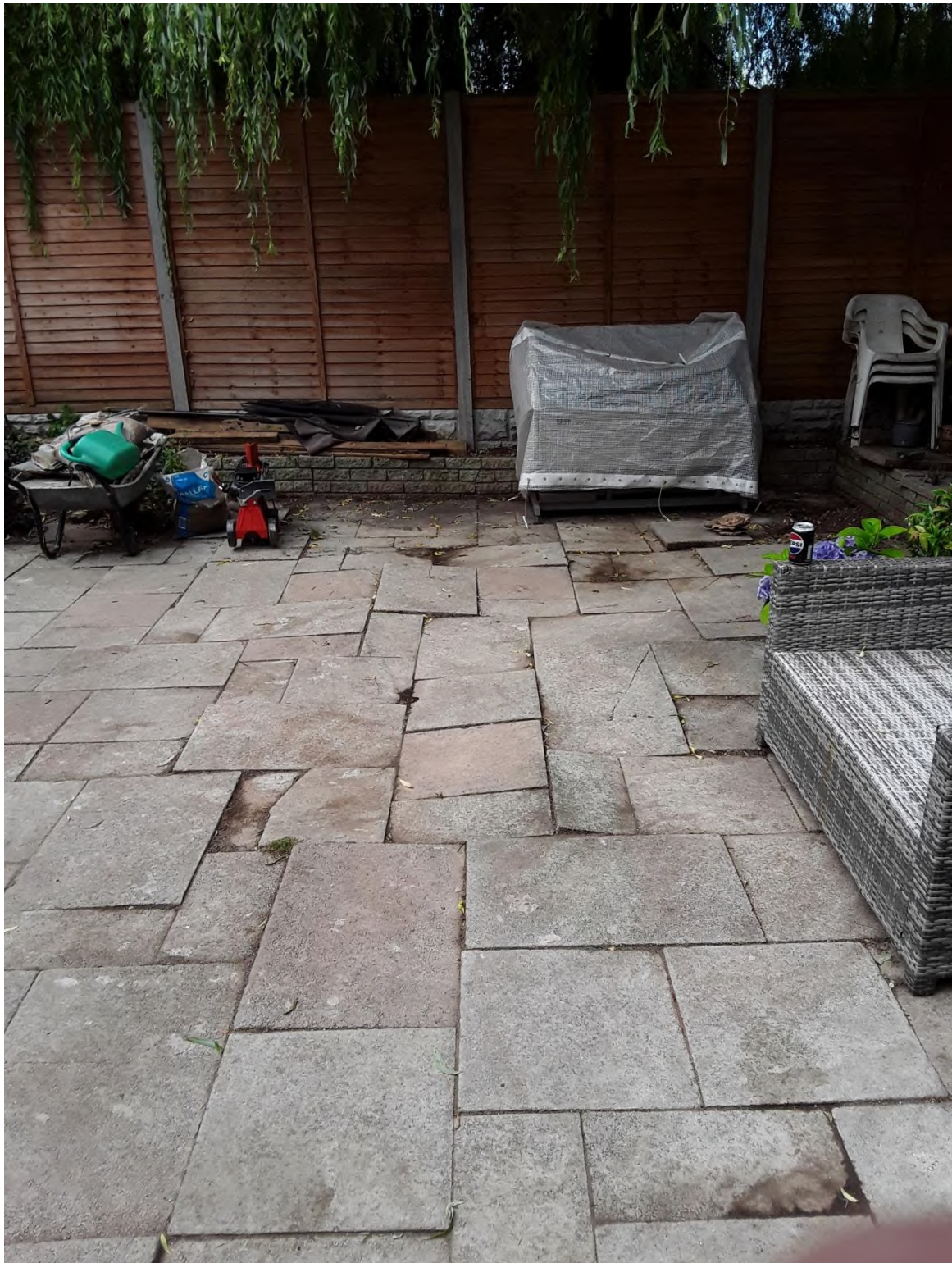
Image 11 – Dislodged patio due to tree root damage
