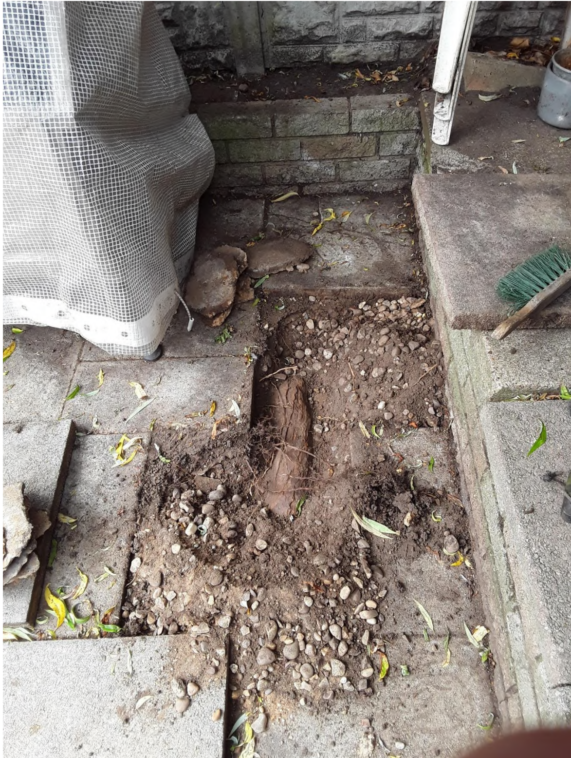
Image 10 – Roots just under patio in rear garden
