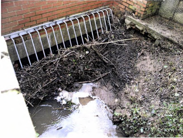
Document 3 – Photograph of Culvert Blocked with Debris
