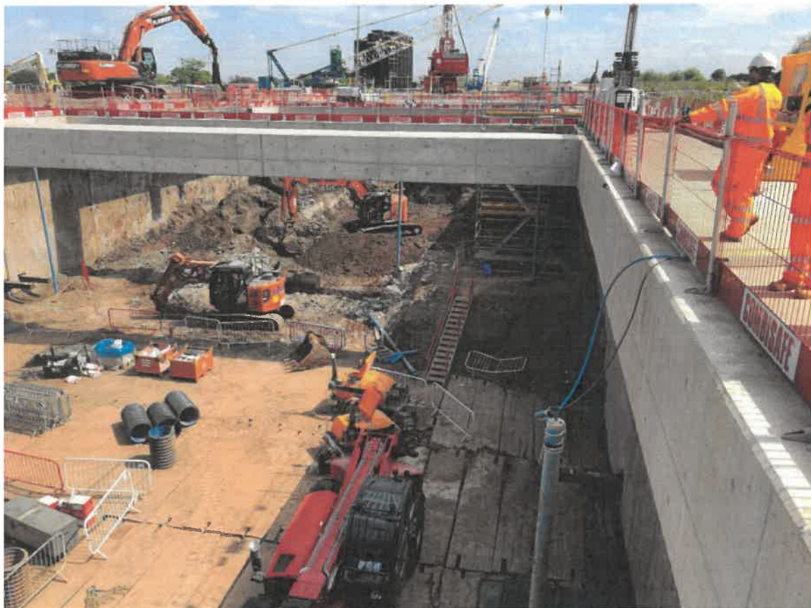
Water Orton Cutting looking eastwards, west of the cutting's merging with the proposed relocated tunnel portal
