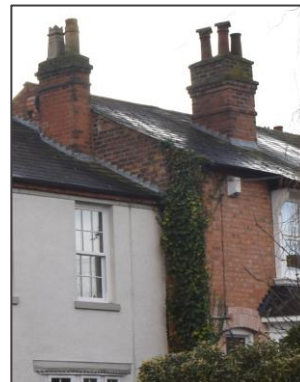
Ivy growth at Albion Terrace
