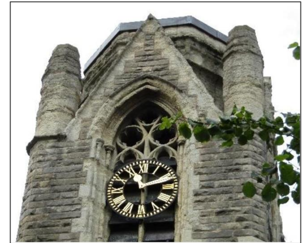
Sandstone detailing eroding at St Peter and St Paul Church
