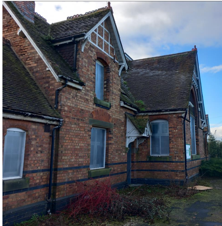
Former Primary School now boarded up, still being entered by vandals causing damage to the interior and roof.
