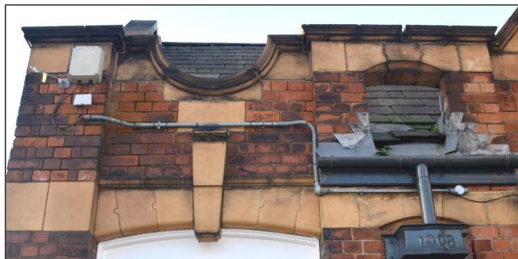
Faience (glazed terracotta) used in the Train Station as a decorative, but affordable material.
