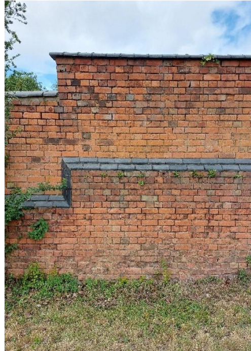
The brick garden wall to the Hall kitchen garden is constructed in England bond (alternating beds of headers and stretchers). By making the wall thinner halfway up its height, it could be built without the need for buttresses or piers. The blue clay copings to the lower and upper sections of wall help to keep the brickwork dry.
